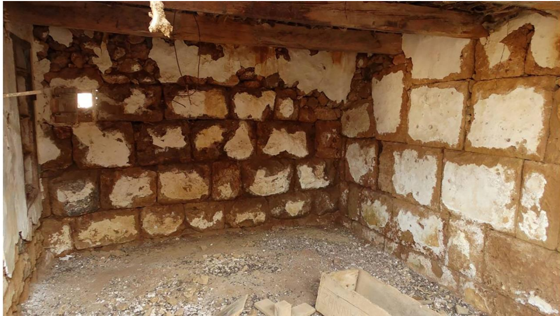
Fig. 7 House of the 19th century where the ancient fortification wall was used.
